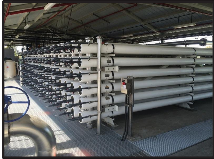
Figure 3 Primary RO Train
