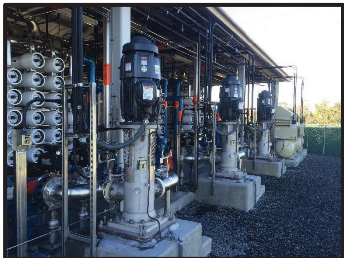
Figure 6 Concentrator RO Trains
